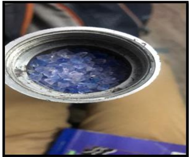
Figure 4: Opening for maintenance of silica gel
